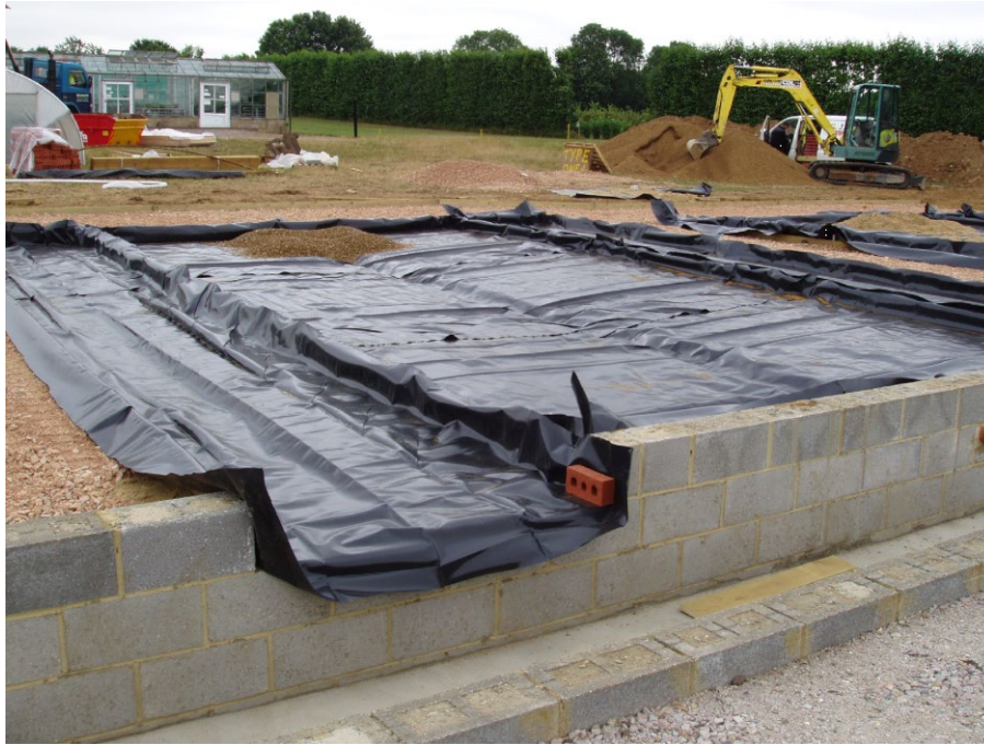
Figure 8: Laying the water collecting polythene under the capillary bed and waste water collection areas, left and right of the main bed, at the East Malling Water Centre. Waste water missing the bed, when sprinklers are in operation, is collected in the waste overflow drain as seen on the left
