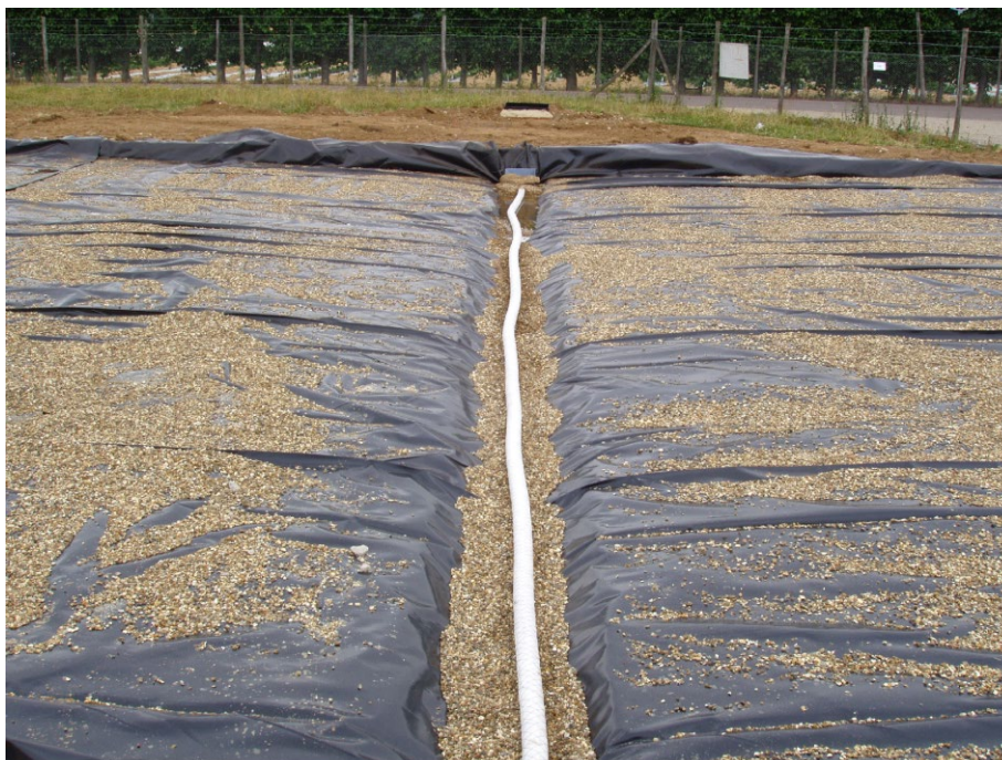
Figure 7: Main drain of the large overhead sprinkler (10 x 30m) gravel bed at the East Malling Water Centre. The central rapped drain pipe is shown along the bed length
