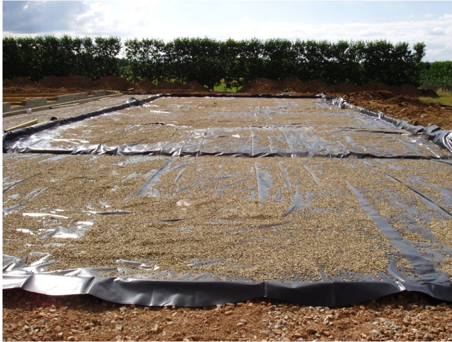
Figure 6: Construction of the large (10 x 30m) overhead sprinkler gravel bed at the East Malling Water Centre. The bed is sloped from left to right and contains two main drains
